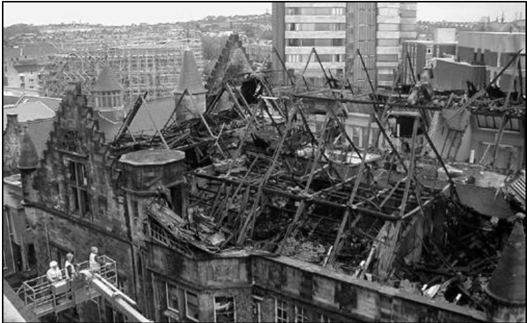
Figure 2 Bower Building, University of Glasgow. 24 November 2001. Category A Listed building extensively damaged with an estimated £7 million loss. Many historic books also lost. Cause unknown, but thought to have started by fireworks.
