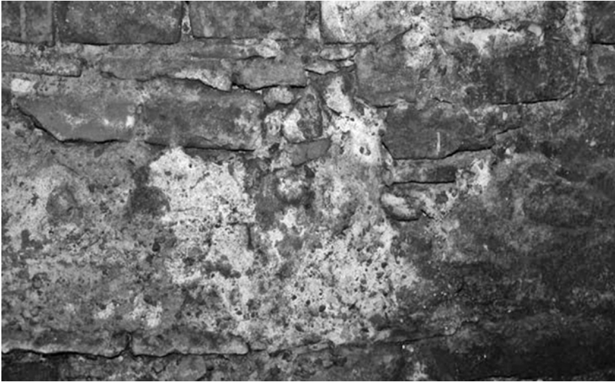
Figure 3 Salt efflorescences related to a soot cover generated by fire (picture courtesy of Mr P. Rohlen)
