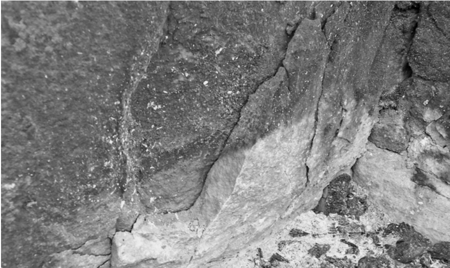
Figure 2 Sandstone after a localized fire at Dungiven Priory, Northern Ireland – note the discolouration (reddening) of stone in the ‘clean’ area where the flames burned, the soot-coated stone above, and the fracturing which caused severe loss of material.
