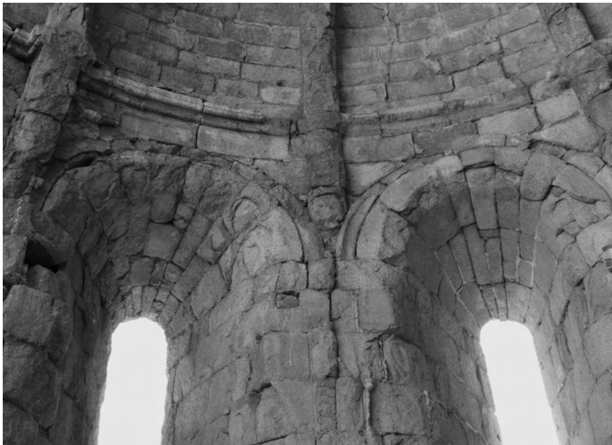
Figure 1 Severely spalled granite as a consequence of an historical fire. The concentrically ‘onion-skin’ structure of the spalling is especially noticeable in the window arches, through which flames may have moved to the exterior of the building.
